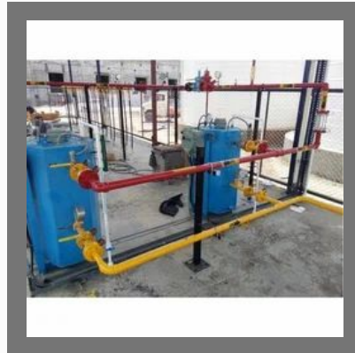
Pre Piped Gas Trains
